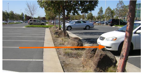
Figure 5-14: Failed pedestrian circulation within a parking lot. Due to poor design, people have trampled this vegetated swale to the point where the landscape cannot grow.
