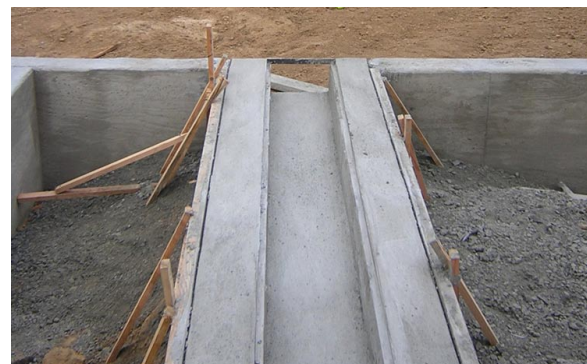
Figure 5-55: Hardscape elements, such as this trench drain channel, should be inspected to ensure positive drainage into the stormwater facility.
